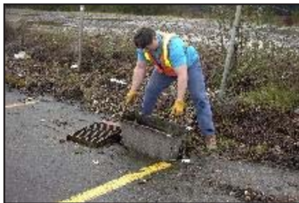
Figure 7. Maintenance of a bag type water quality insert. (Filter Bag Installation (Full Circle Ag, Inc., http://www.fullcircleag.com/pages/954364/ ))
